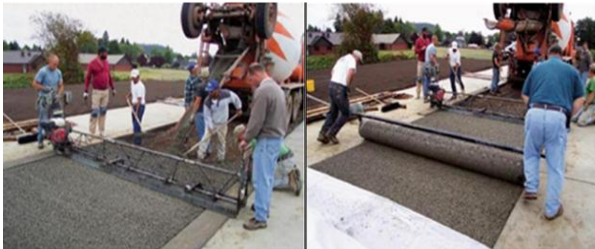
Figure 2-16. Compacting Pervious Concrete Using Vibratory Screed (Left) and Weight Roller (Right) (Adopted from [54])
