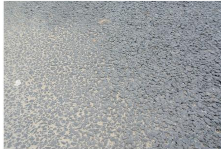
Figure 2-24. Common Clogging Failure Caused by Surface Runoff
