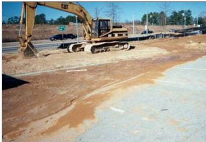
Figure 2-23. Clogging Failure Caused by Construction Traffic
